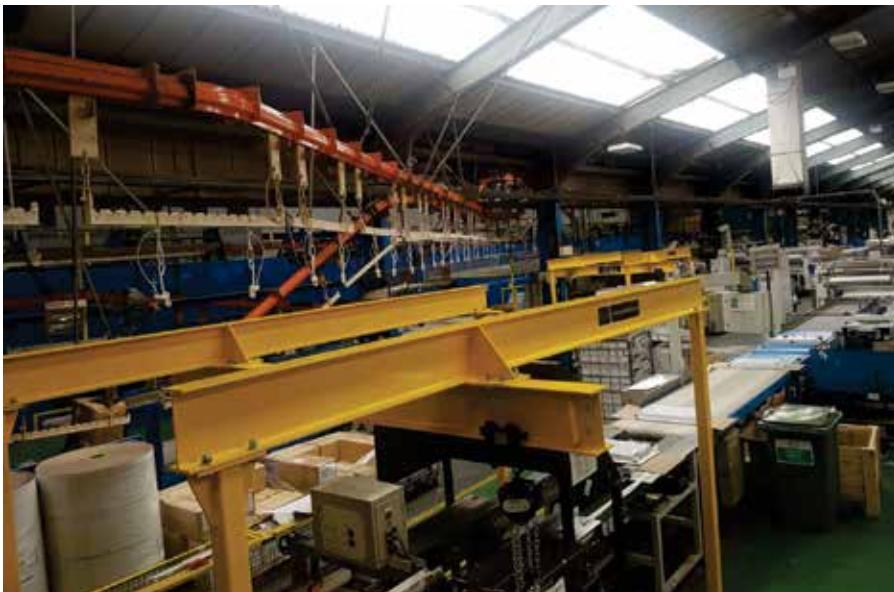
The 500kg safe working load (SWL) goalpost runway systems, installed by Rope and Sling Specialists, span packaging lines at Stelrad's Rotherham facility. The solution eliminates the need for manual handling of heavy parts.
