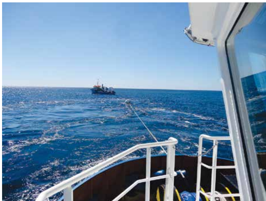
The RLP was used to measure pre-tension up to 30t to check new anchors were properly installed into the seabed.
