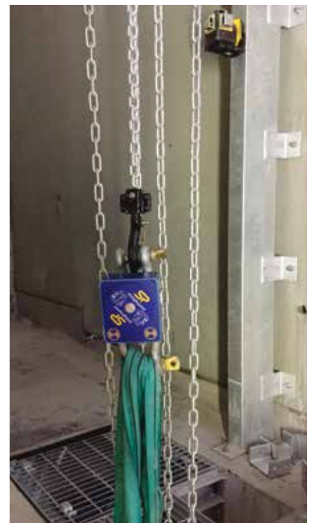
HES used a proprietary surface-mounted test rail that was rigged up using synthetic slings.
